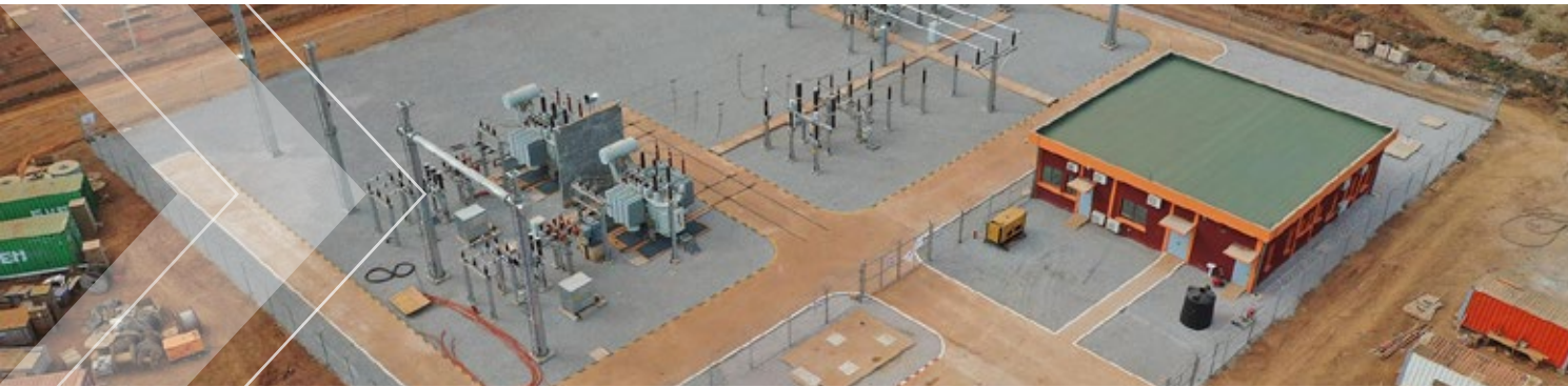
High voltage substation at Séguéla Project
